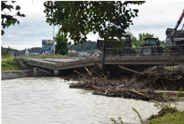
Figure 2. Partly collapsed bridge after floods (upstream).
